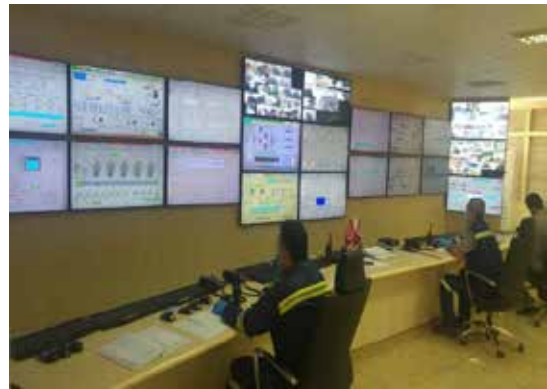
Figure 3. Central Control Room
