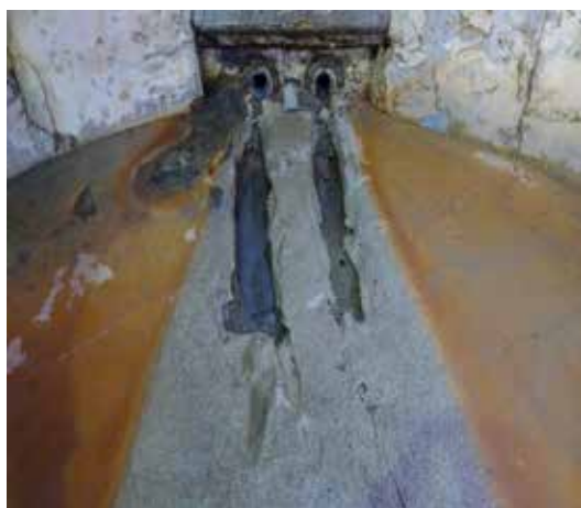
Figure 4. Granulated Inba Inside Chimney Floor Wear
