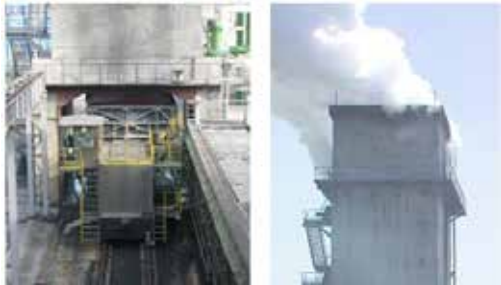
Figure 2. Wet Quenching System
