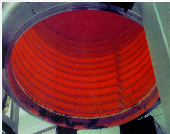
Figure 5. View inside an electrical Heating Hood with resistance heating system.
